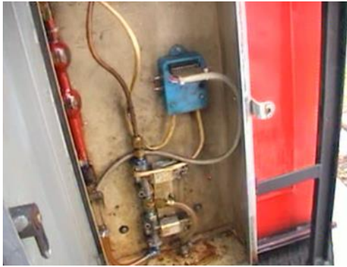
Fig. 3. View of the fuel metering unit in the tow truck
